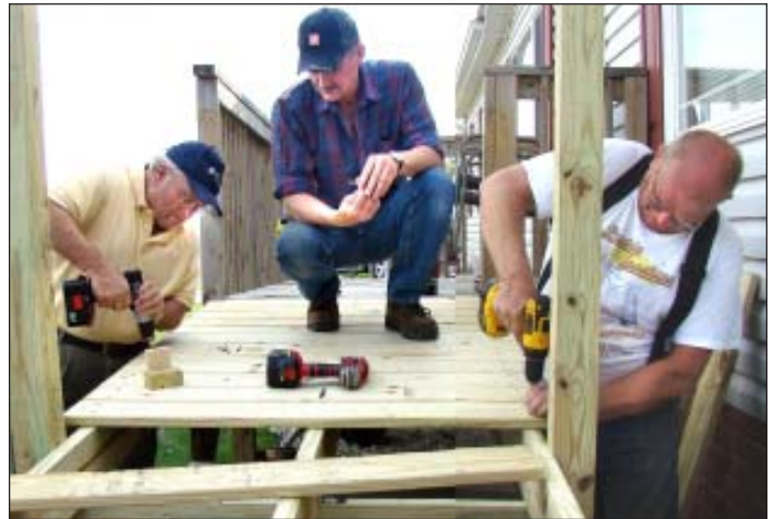
The Jacksonville Ambucs service club construct a ramp on the east side of Jacksonville.
